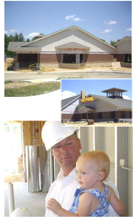
Good Shepherd in Midlothian VA recently held their first "hard hat walk through". Even the youngest attendees were impressed with the new facilities being constructed..
