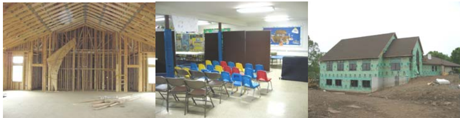
The members of St. Peter Lutheran Church are excited to visualize their expansion project.
